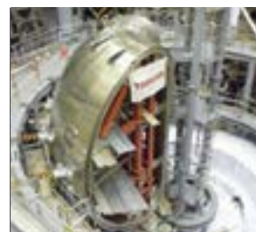
Fusion Reactor Vacuum Vessel (JT60SA :JAEA)
