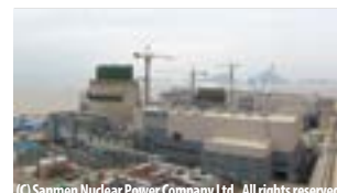
AP1000™ Next Generation Pressurized Water Reactor (Sanmen Nuclear Power Station unit No.1 : SNPC)
