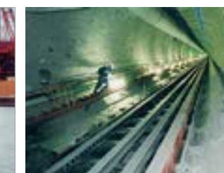
Kannagawa hydropower station
