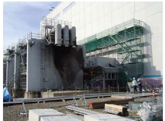
The transformer of the unit-3
