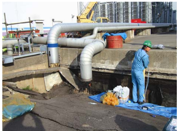
An area where the ground subsided by approximately one meter. Within the NPS's perimeters, interim restoration work has been done on the roads, making them passable, but even now, work to repair ground subsidence, etc., on the roads is taking place everywhere.
