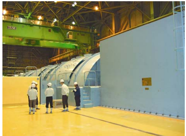
An earthquake meter (lower center) in the upper part of the turbine mount of Unit 3, which experienced the greatest earthquake acceleration in the July 16 quake. The acceleration experienced was measured at 2,058gal (in an E-W direction), some 2.5 times the design acceleration of 834gal.
