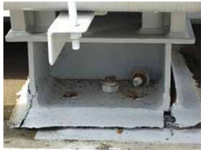
Anchor bolts of main transformer, Unit 2 (C)
