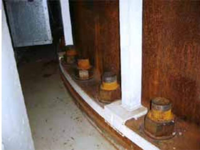
Anchor bolts for RPV, Unit 1 (As)
