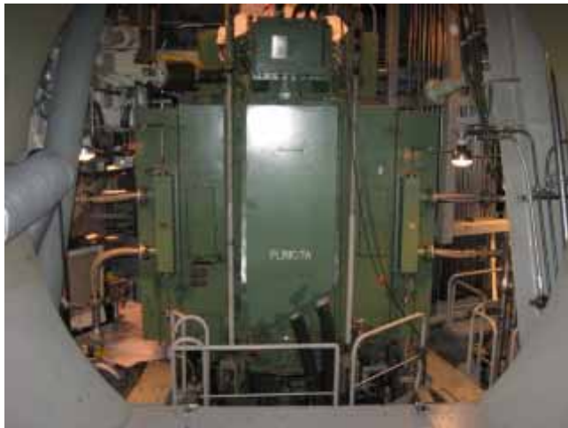
Primary loop recirculation. Pump, Unit 1 (As)
