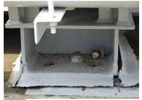
Damaged anchor bolts for transformer (C)
