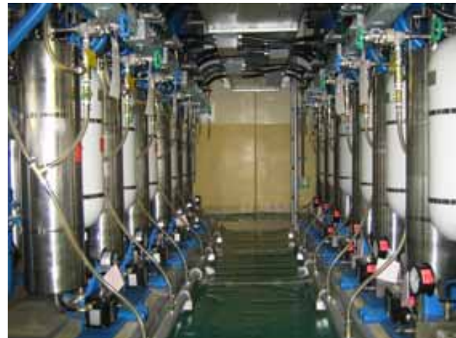
Pressure control unit, Unit 1 (As)
