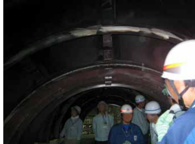
Inside turbine cabin, Unit 1 (B)
