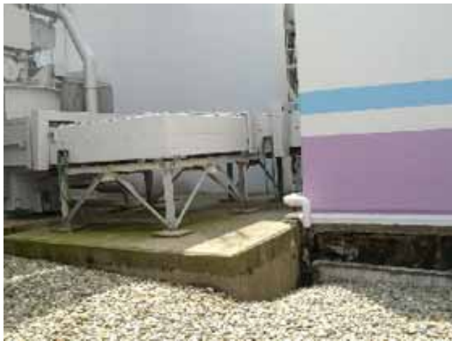
Ground subsidence, Unit 2 (-)
