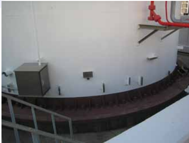
Fuel tank for emergency diesel generator, Unit 1 (C)
