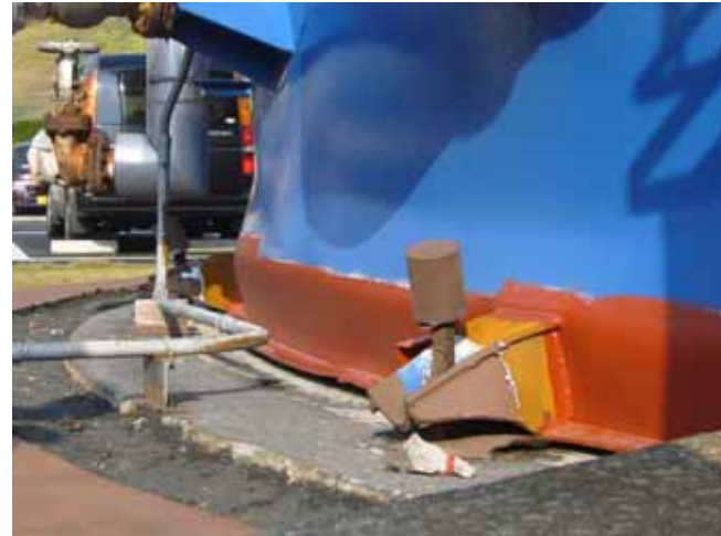
Filtrate tank, Unit 4 (C)
