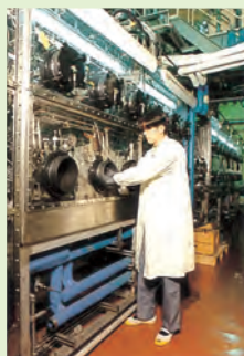
A tritium handling system with glove box
