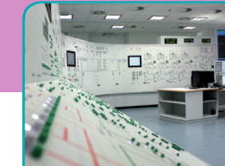
4 Control room with advanced digital I&C systems
