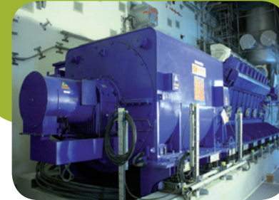
Emergency diesel generators
