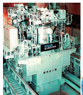
Ex-vessel fuel transfer system
