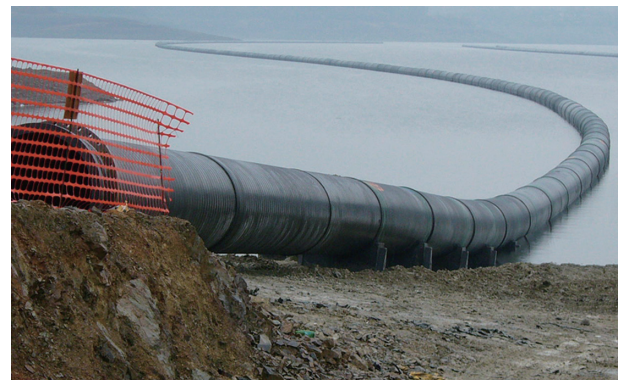
Seawater Intake Pipe
