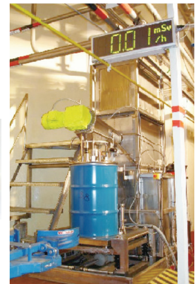
Example of SIAL® Pre-treatment facility (Courtesy of Wood)
