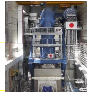
NBTF: High Voltage Tests for JA components completed (Nov 2019)
