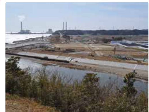
楢葉町で建設中の海岸堤防 New sea embankments being built in Naraha Town
