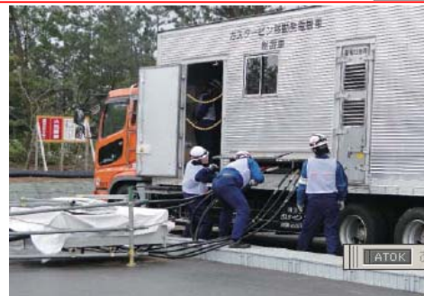
On board Gas Turbine Generator (4500kVA)
