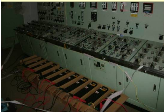
Car Batteries connected to the Instruments Panel
