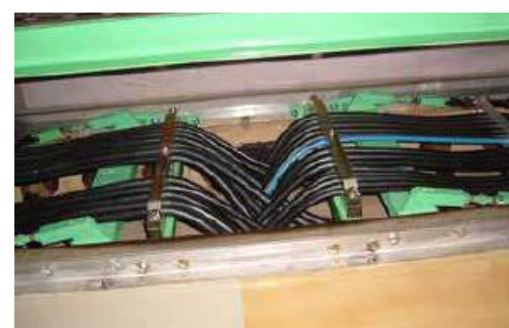
Cable Junction Box
