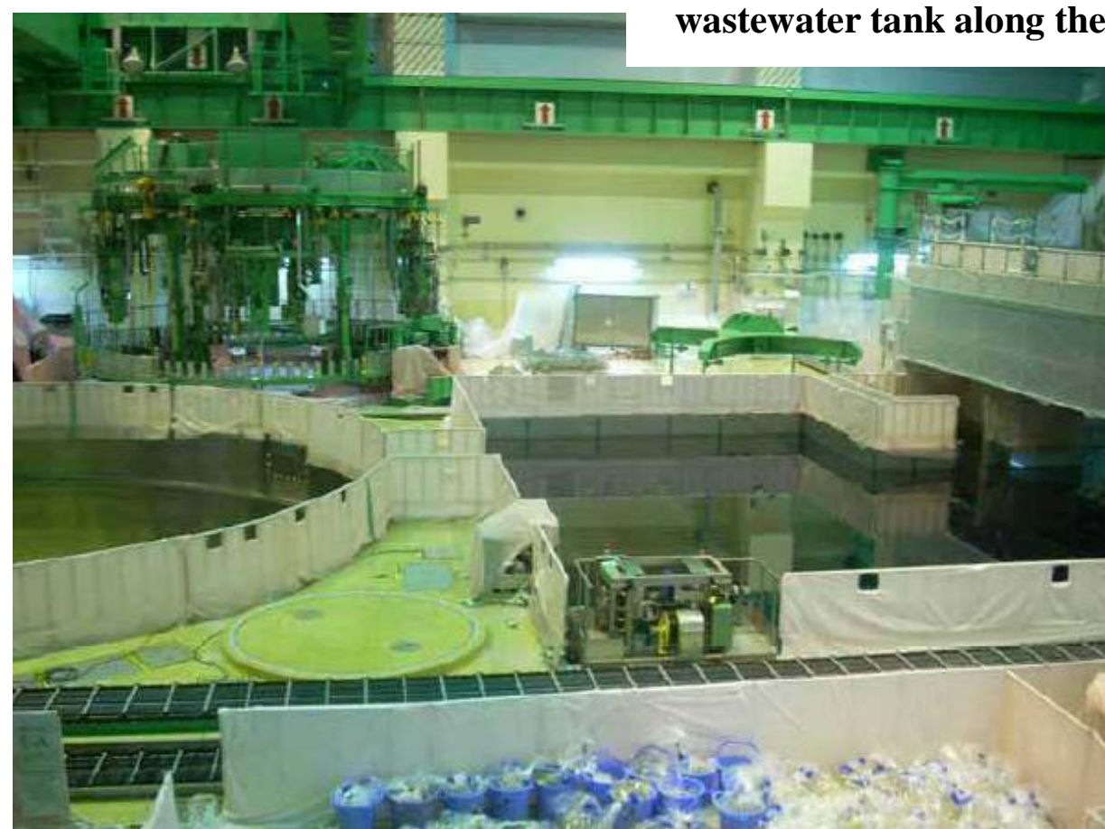
Overview of Operating Floor
