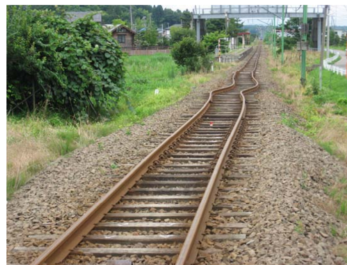
Railway was bent
